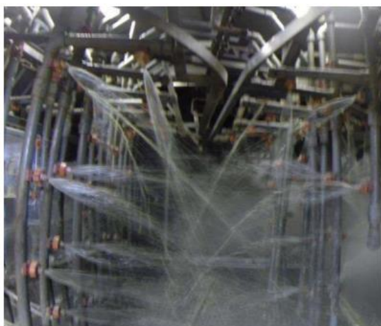
Extremely poor spray pattern
