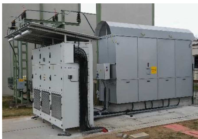
Fig. 1. Final STATCOM installation in distribution power grid of 22 kV
